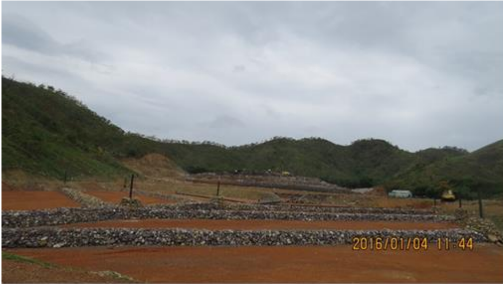
The almost Completed fish bone structure (Cell 1) supplemented with rock covering and extended vent pipes
