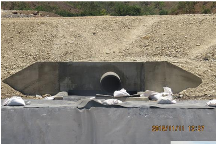
End of main leachate pipe
